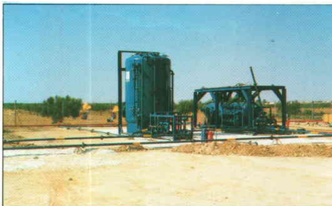
Surge tank and Gas Oil Separator for SLK-1 oil production in Tunisia
