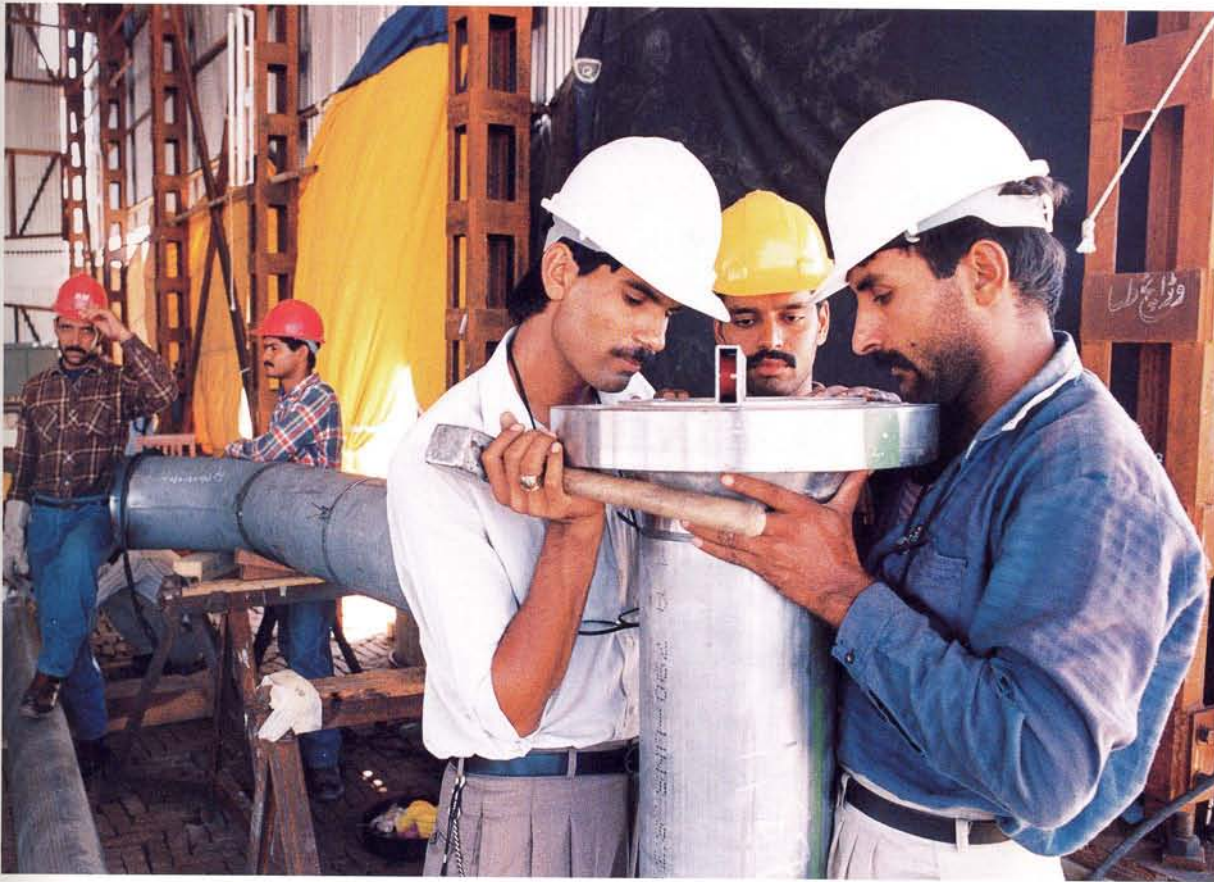
Pakistani workers adjust a flange on the Kadawari gas plant. As early as 1983, discussions had been entered into with the Pakistani government to acquire a concession for which KUFPEC hoped it would be operator. It was a number of years before the negotiations were successfully concluded, but the path to operatorship was being built.
